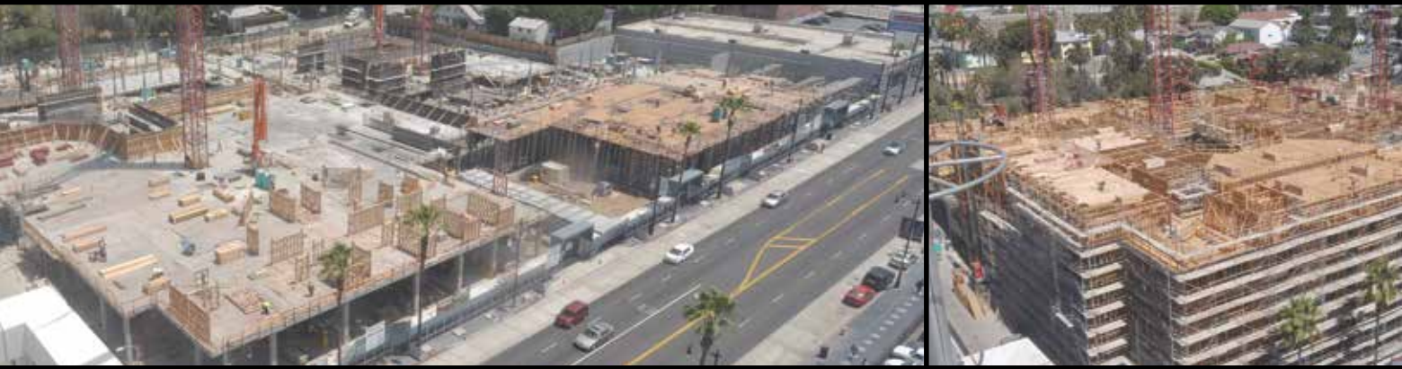
Photos 2-4. In this 500-unit project at the intersection of Hollywood and Vine, the builder saved $300,000-400,000 in construction
