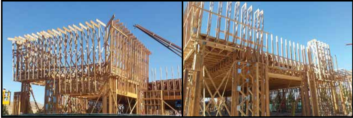
Photo 1. The builder completed this 5,000 square foot commercial mall project 30 days earlier than planned and saved $80,000.
